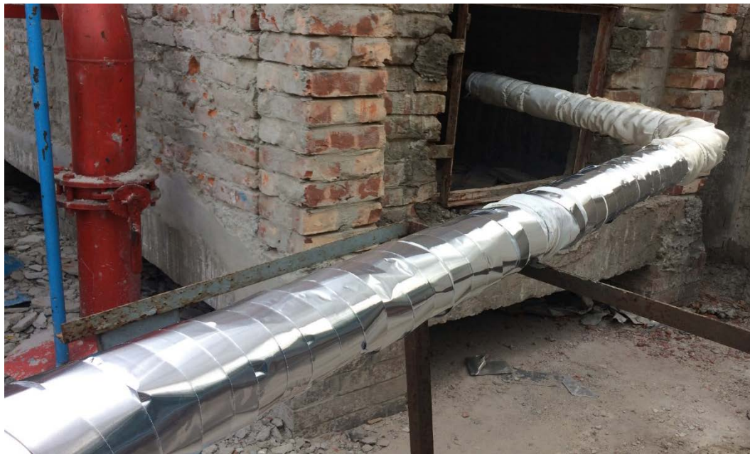
Figure 4.4: Triple layer Insulation over Iron Pipe.
