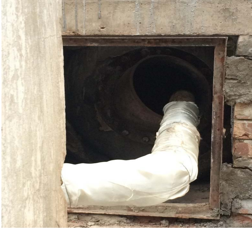
Figure 4.3: Taking Exhaust Gas from the Engine Chimney.
